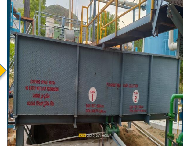
Flush out storage MS tank
